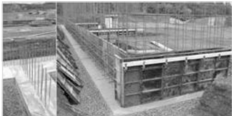
Construction of the new Highway Salt Barn: footers completed (left) and formwork for walls (right). Photo: Ted Crane
