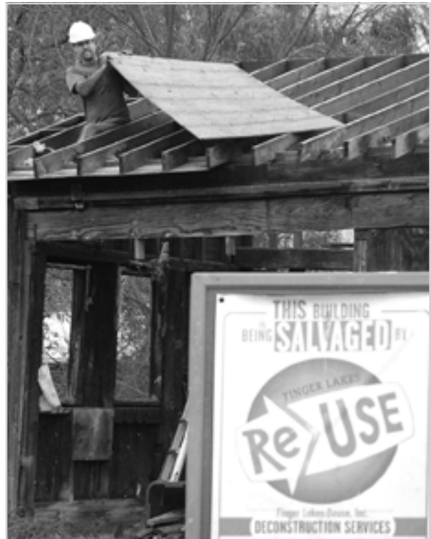
Old House Being Recycled Into New Alex Soule's aged garage wasn't always at the corner of Danby and Bald Hill Roads. Before Ed Slaights moved it, it served as a blacksmith's shop! Now it's being deconstructed by Finger Lakes Reuse, who will sell its parts for use in new construction. Check out [fingerlakesreuse.org]. Photo: Ted Crane
